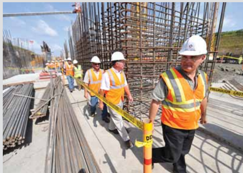
Members of the Canal Board of Directors inspect the Pacific lock site.
