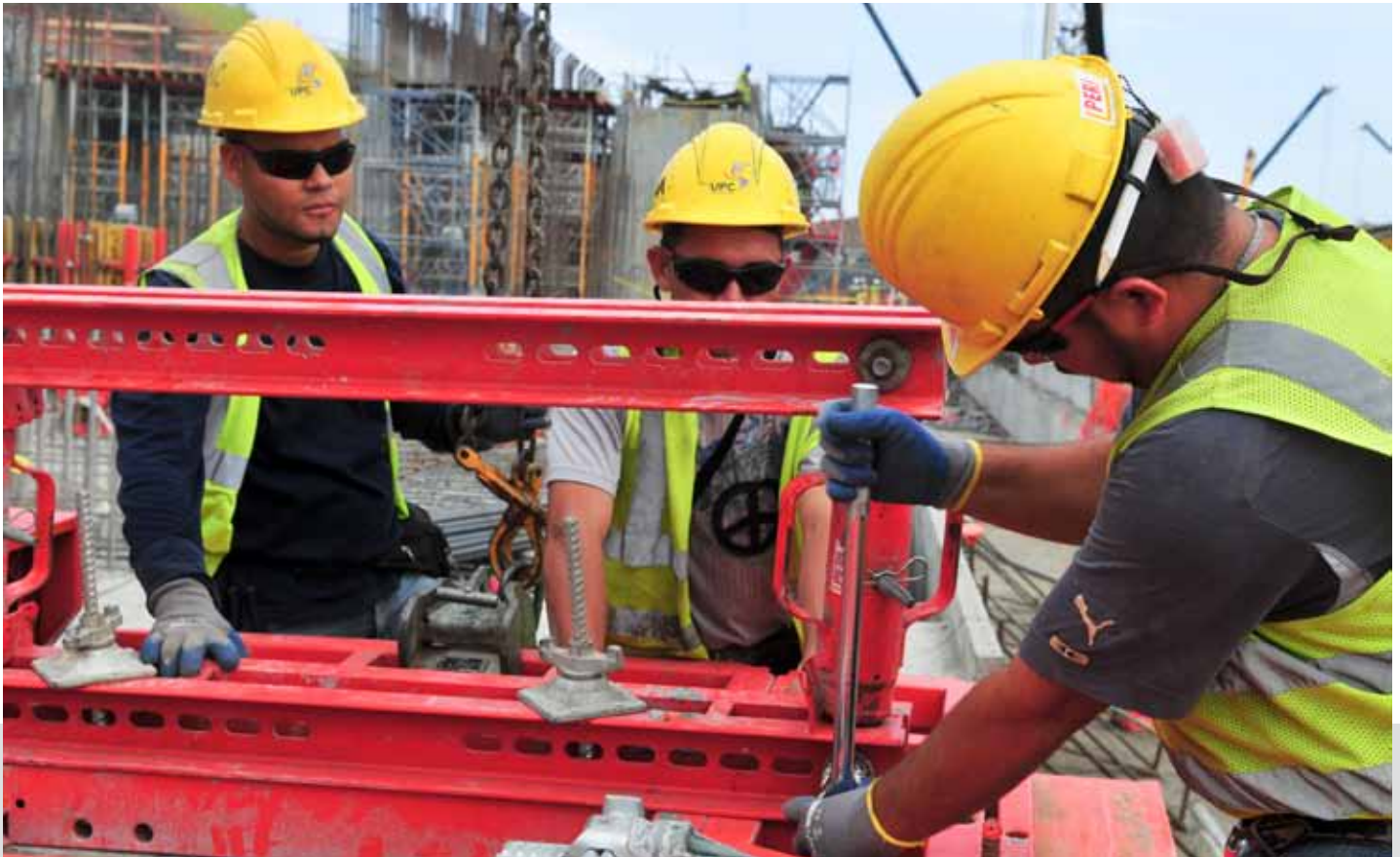
Installation of form work for concrete pouring activities at the new Pacific locks.
