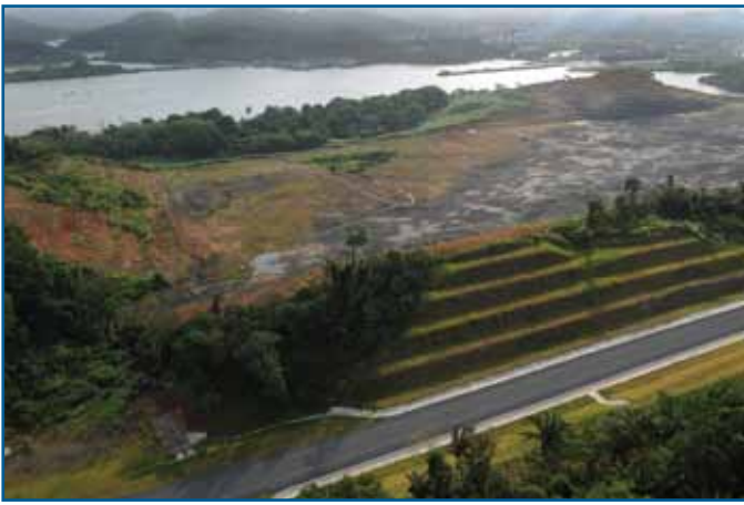
The new Borinquen Road. Work under PAC-2 is seen in the background.
