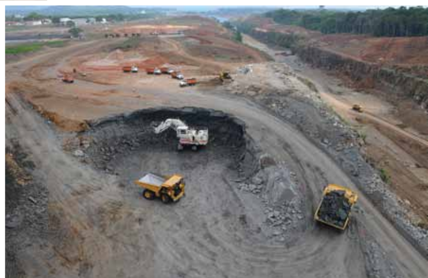
Large heavy equipment is used to conduct excavation work on the Atlantic side.
