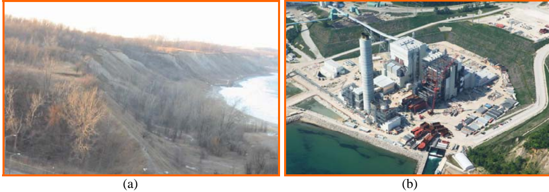
Figure 1. Construction site along the shoreline of Lake Michigan: (a) before excavation; (b) during construction.
