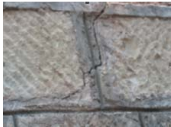
Fig.5 the cracked retaining wall
