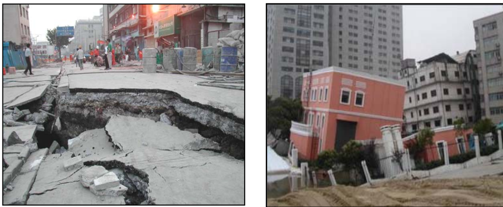
Fig.3 Crack of adjacent road and inclination of the adjacent pump room
