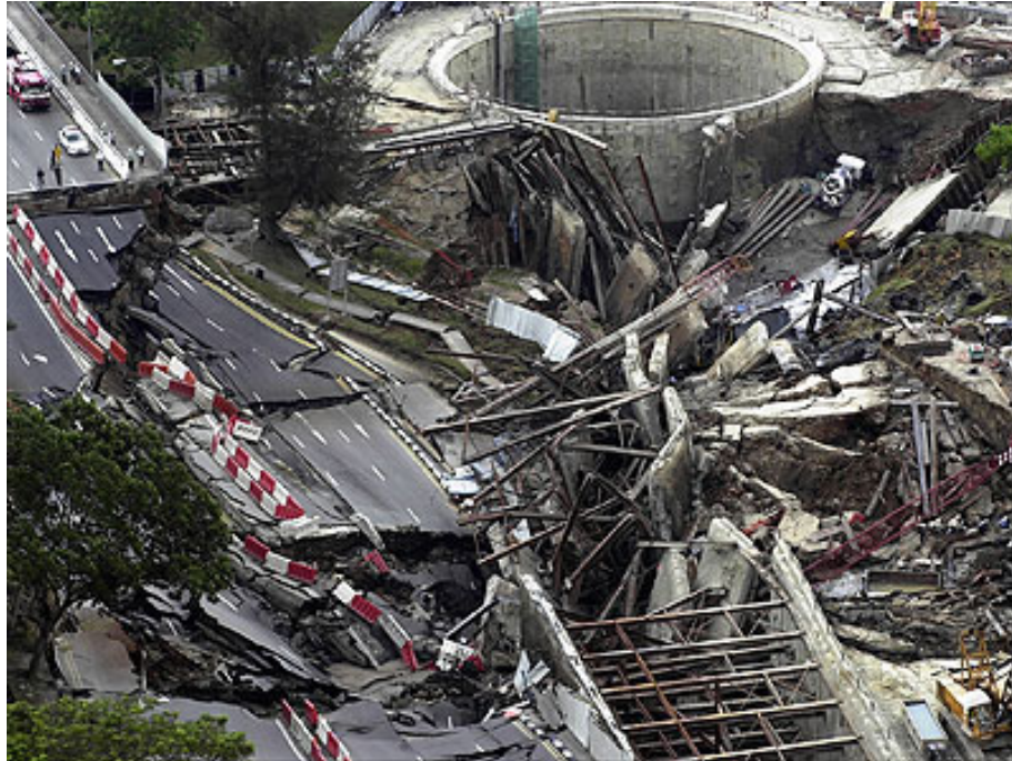
Fig.1 Nicoll Highway deep excavation in Singapore just after collapse on 20 April 2004
