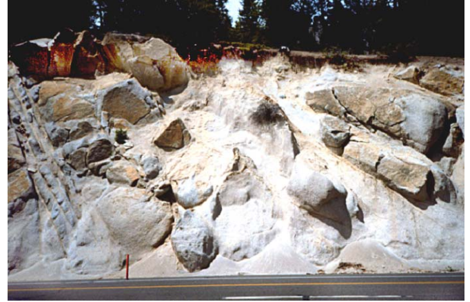
Figure 7. Decomposed granite located in the Sierra Nevada mountains of Northern California. Hard blocks (corestones) surrounded by matrix of “gruss” (granite decomposed to dense sandy soil).
