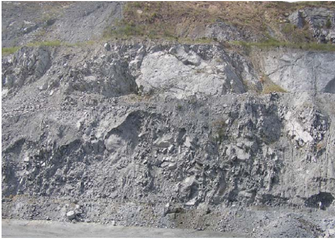
Figure 8. Rock exposed in slope excavated within San Andreas fault zone, Northern California. Sheared rock surrounds hard blocks of relatively intact rock. Blocks range between centimeters to tens of meters in size. (Photo: E. Medley/Geosyntec Consultants).
