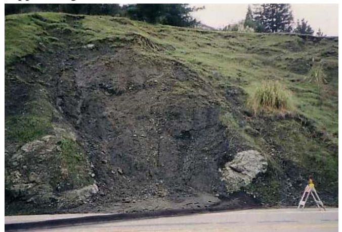
Figure 4. Blocks in Franciscan melange buttress slope between landslides in sheared shale. (E. Medley/Exponent)
