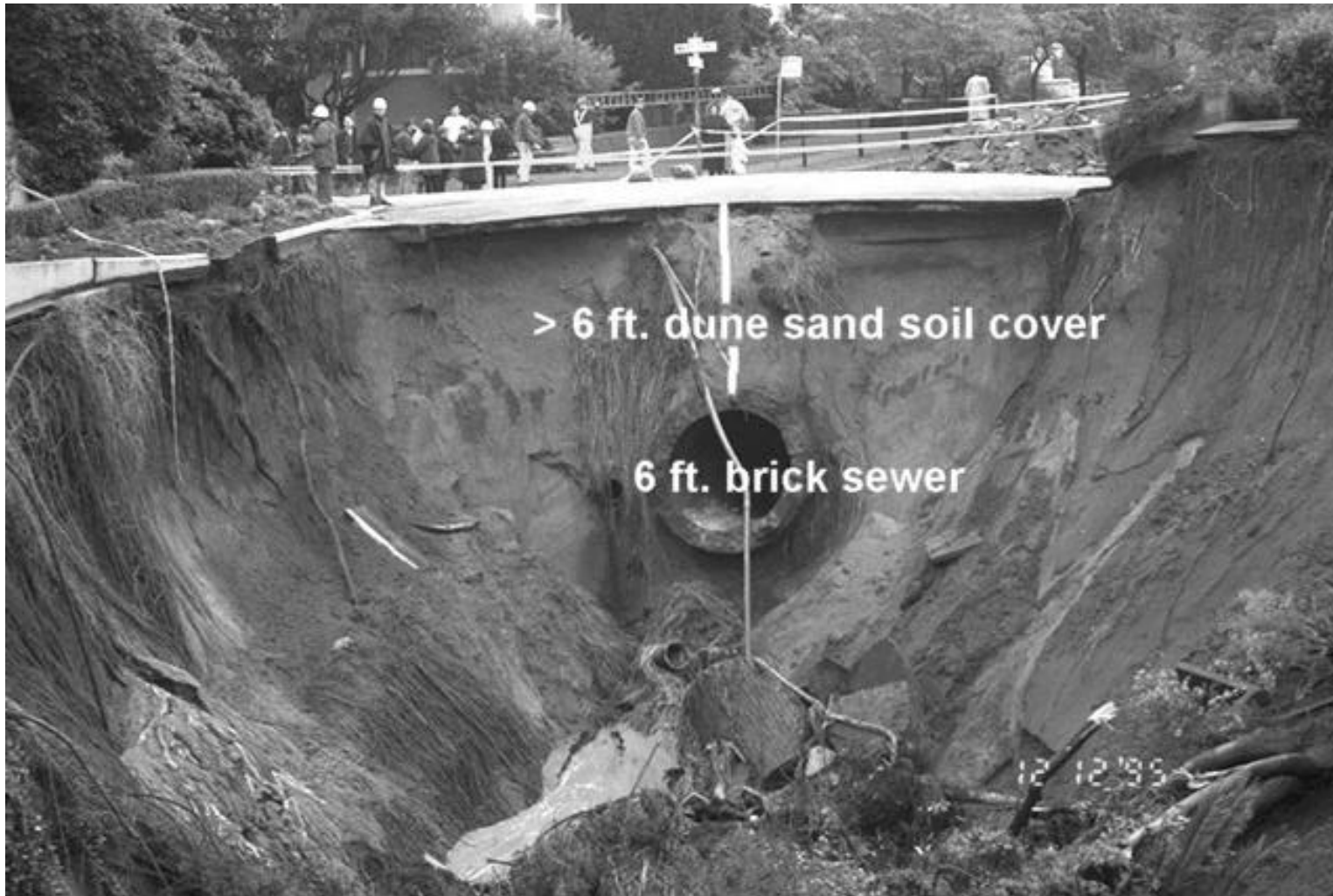
Figure 3 – Remnant of 6-foot diameter brick sewer at the southern limit of erosion. Sewer is confined by loose to medium dense dune sand.
