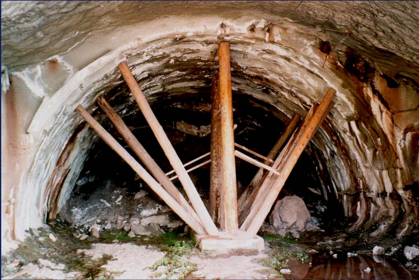
Collapsed Tunnel M2, Egnatia Motorway, Greece
