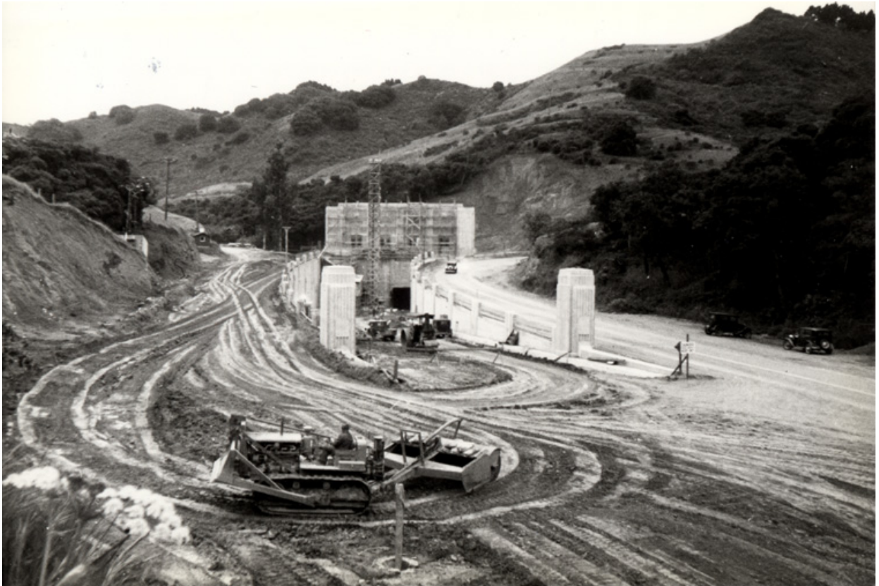
Figure 4. Photograph of the Caldecott Tunnel under construction in the 1930s (photo provided by Caltrans).
