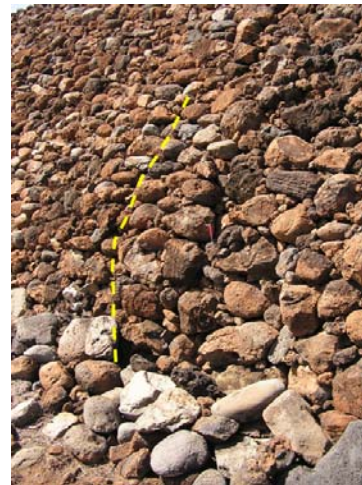
Figure 18. Post-earthquake photo near NE corner of Pu'ukoholā shows bulging of face of wall (indicated by yellow line).
