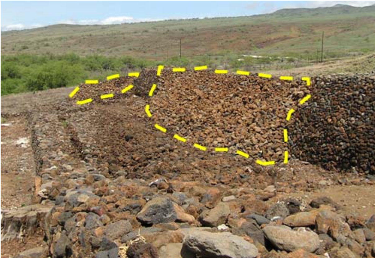
Figure 14. Raveling and slumping of eastern wall of Mailekini Heiau, after earthquake.
