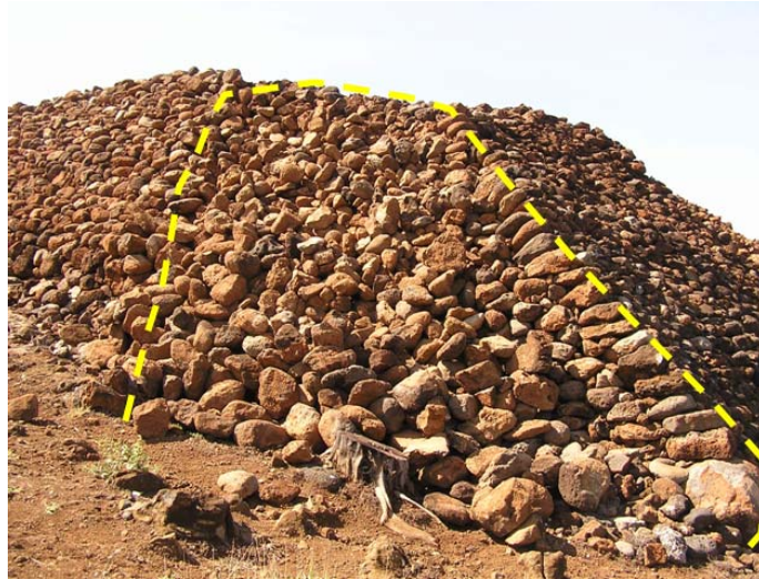
Figure 19. Pu'ukoholā Heiau. Slump failure due to earthquakes (between dashed lines).
